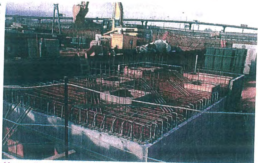
Above, the Vortechs® cast-in-place System during construction. Each of the roof slabs for the cast-in-place units include a steel cross beam to help meet the loading specifications.
